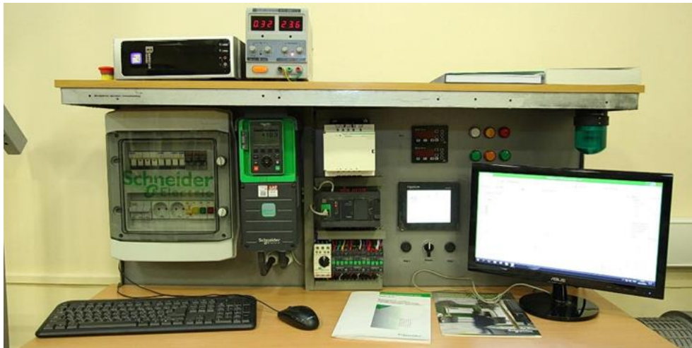
Figure 8. Electric drive SCADA system in university scientific laboratory.
