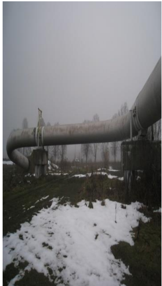
Fig. 1. The plot of the gas pipeline from the transition of underground laying in the ground. (gas pipeline Urengoy - Pomary - Uzhgorod)
