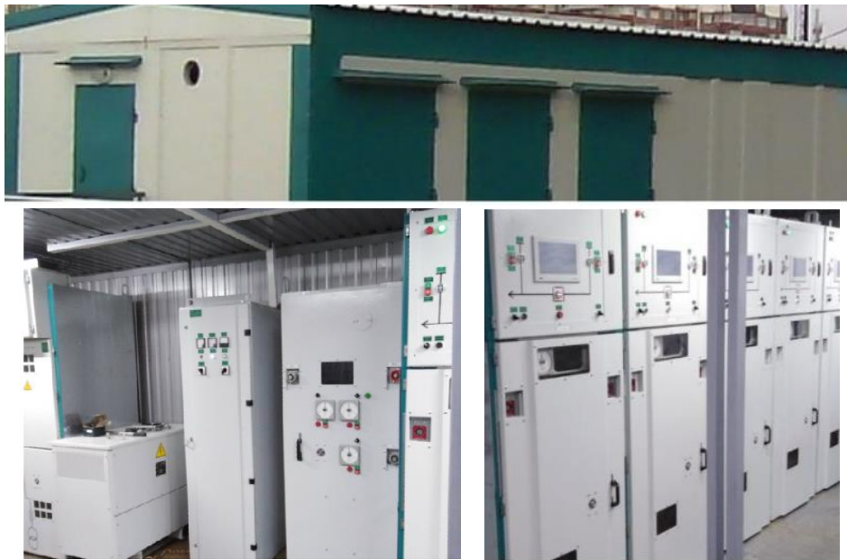
Fig. 3. Modular design traction substation of urban electric transport TIIM-MT-3-1000-6/600 in Kharkiv
