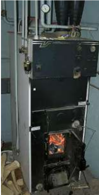
Central heating unit.
